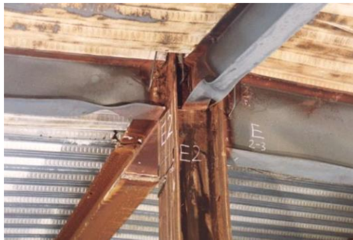
Figure 4: Steel warped after being exposed to high temperatures from a fire
