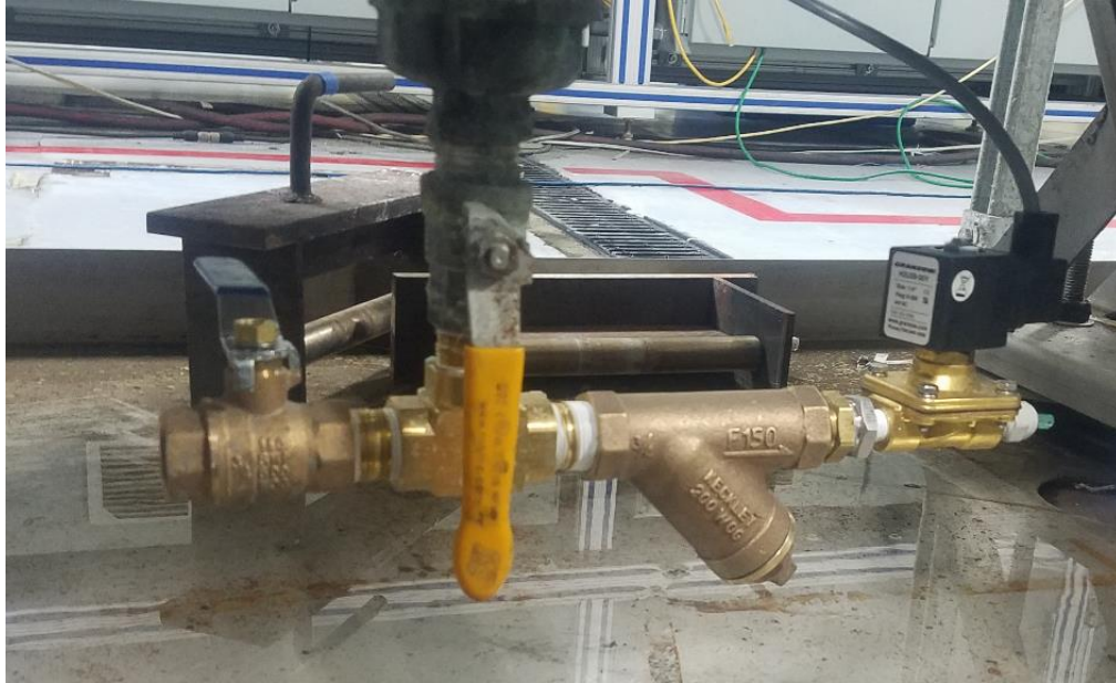
Figure 13: The valve assemble in place on the assembly line.
