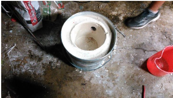
Figure B2. The forge after the fire concrete has cured for 30 minutes and the air supply hole has been drilled and the plastic bucket has been removed.
